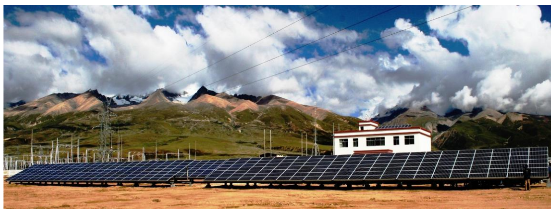
Figure 9 LSPV Grid Connected PV Pilot System in Yangbajing of Tibet, 100kWp
